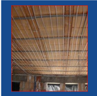
Ceiling Heating System
