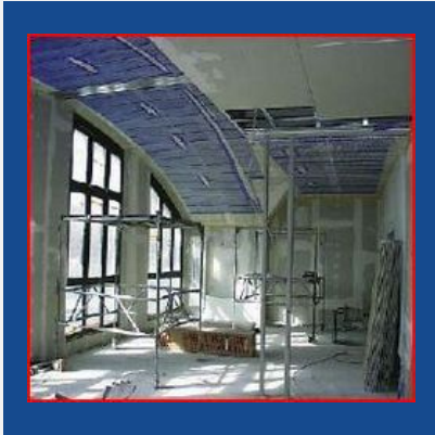
Ceiling Cooling System
