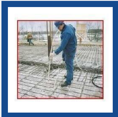
Slab Heating System
