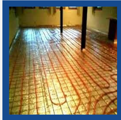
Radiant Floor Heating System
