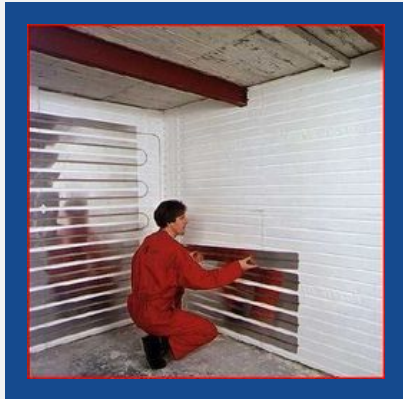
Wall Cooling System
