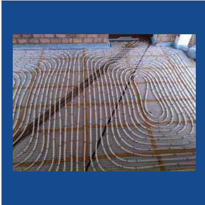
Floor Cooling System
